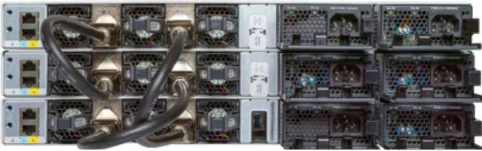
Figure 5. Cisco Catalyst 9300 Series switch stack units
